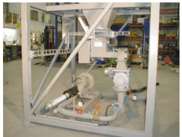
Project Rönnskärsverken in the north of Sweden. Plant for feeding and pneumatic conveying of activated carbon for flue gas cleaning.
